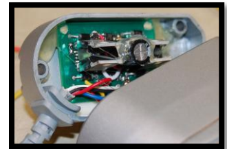
Figure 37. Custom-built motor controller mounted inside the linear actuator. The actuator's limit switches act as sensors for the controller to turn off the actuator motor.
